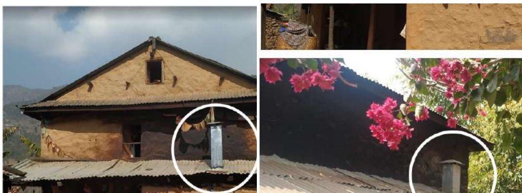
Some installation flaws detected thanks to visual verifications. Currently they are avoided thanks to the location approval step.
