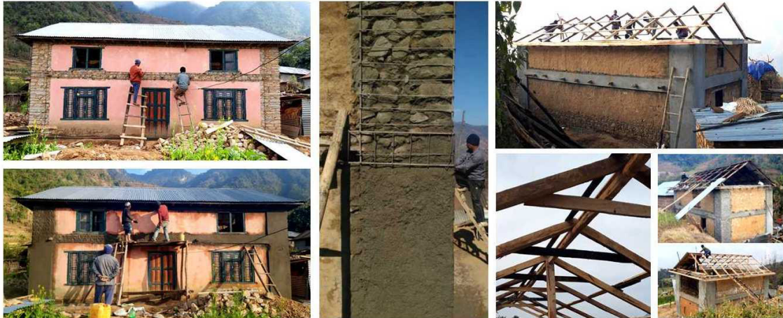
The retrofitted houses almost finished, with reinforced corners and added wooden diagonals.
